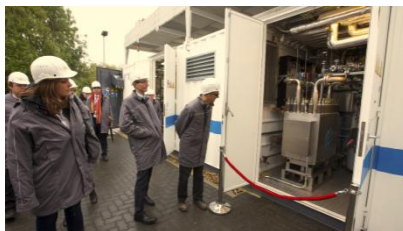
Field test 1.5 MW electrolyser
